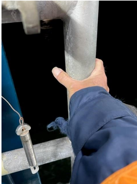
No firm grip, slipping hazard..
